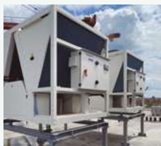
CÉDRUS LIGET, a complex facility including apartments, penthouses and showrooms etc. Hungary. ECOi-W - ECOi - PACi
