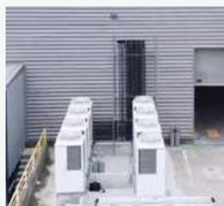
STEMCELL Technologies, a global biotechnology company, installed CO 2 condensing units for cold rooms in the warehouse. France. Refrigeration
