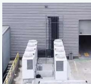
STEMCELL Technologies, a global biotechnology company, installed CO 2 condensing units for cold rooms in the warehouse. France. Refrigeration
